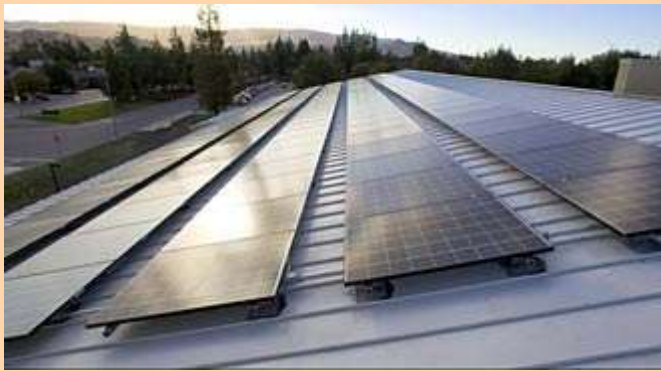
Solar panels atop the Kirsch Center for Environmental Studies
